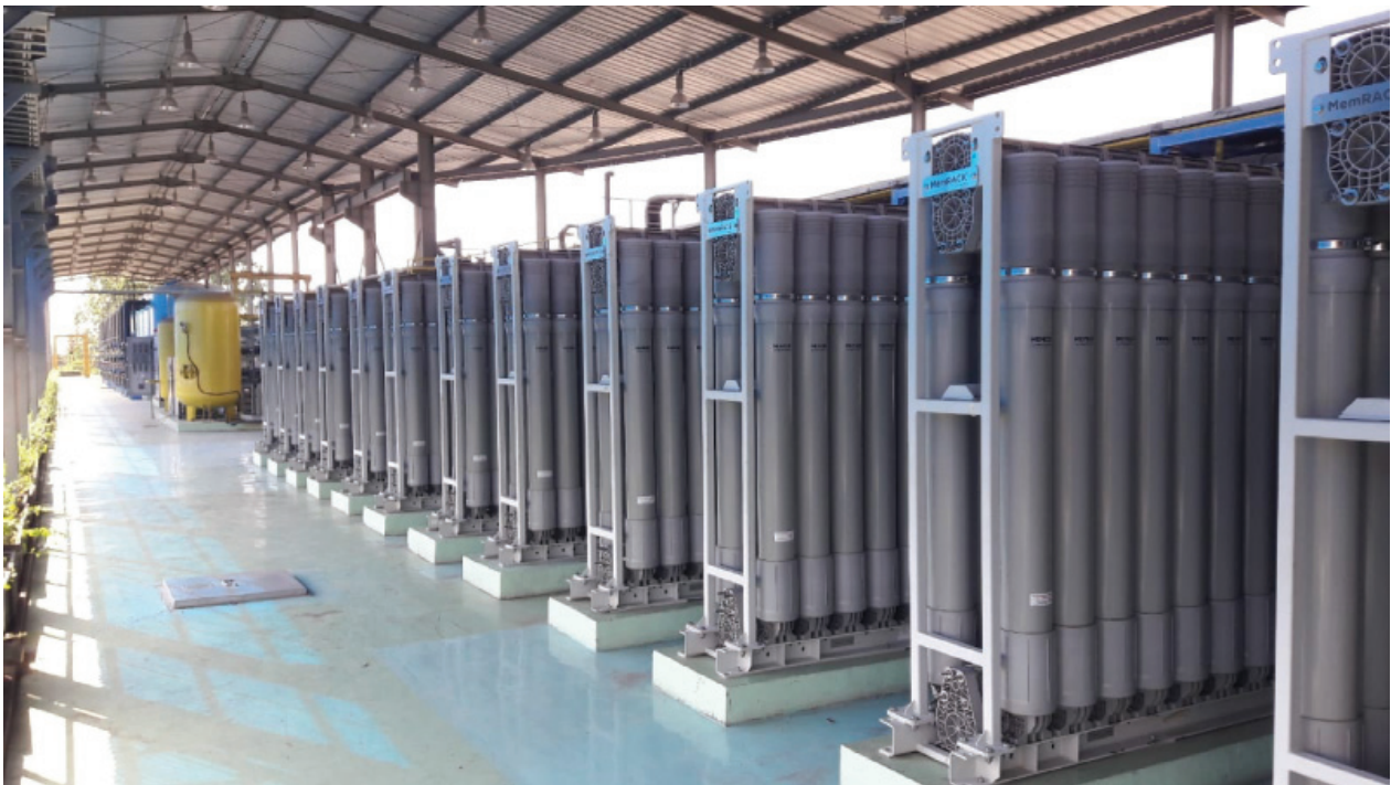
Photographs of the Hutan Kota-located BOOT water treatment plant
