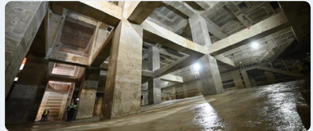
Syed Alwi Pumping Station's underground tank.
