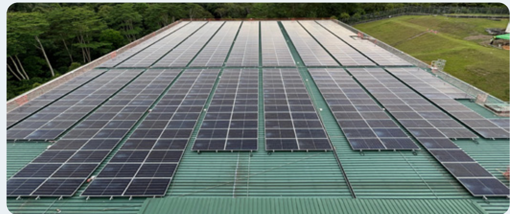
Rooftop solar panels on PUB's premises.
