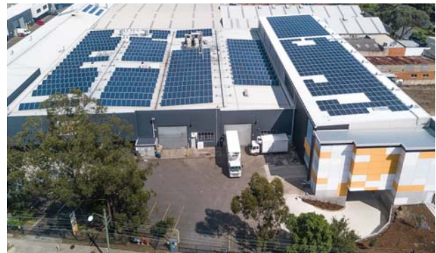
Solar panels installed on the rooftops of BMA's production facility.
