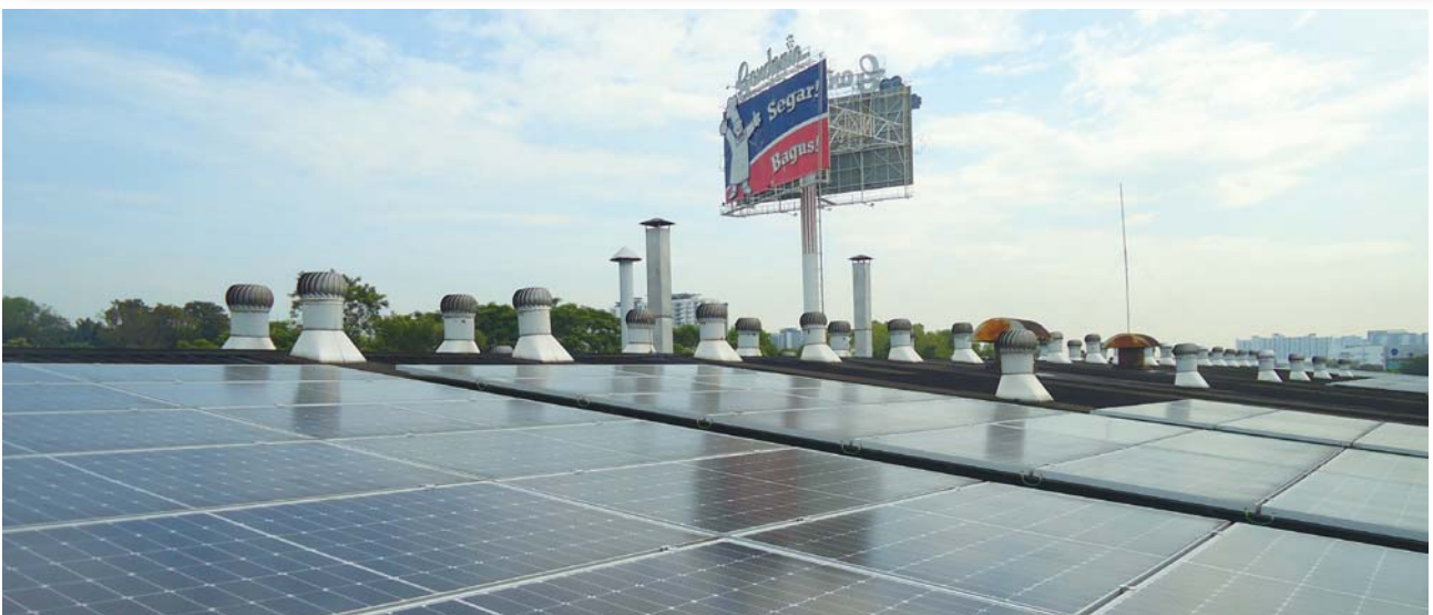
Solar panels installed on the rooftop of one of the factories of our joint venture in Malaysia.
