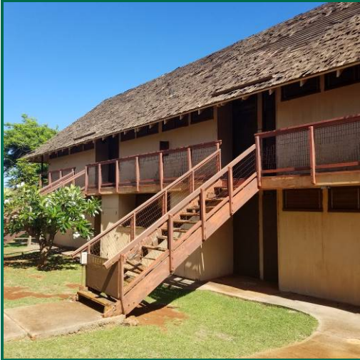
Shuttered Kaluakoi Hotel Structures
