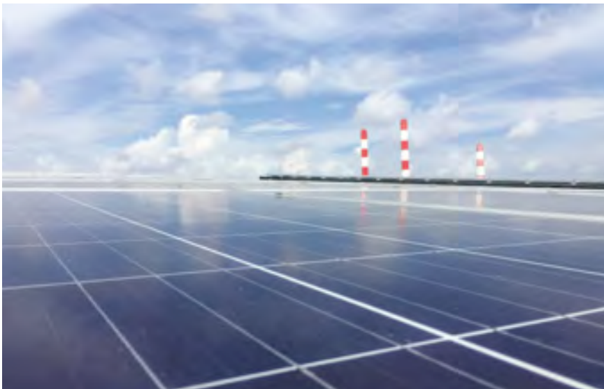
Keppel has announced renewables projects with a total capacity of 1.1 GW, including the acquisition of a majority stake in leading solar platform Cleantech Renewable Assets. (In picture: One of Cleantech's assets in Singapore)
