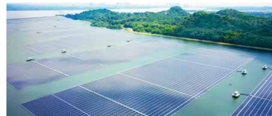
Sembcorp Tengoh Floating Solar Farm in Singapore
