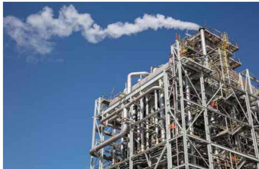
Sembcorp Cogeneration Plant, Sakra on Jurong Island, Singapore
