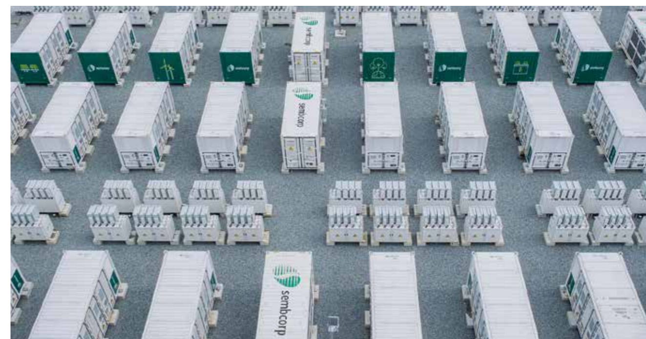
Sembcorp Banyan Energy Storage System on Jurong Island, Singapore
