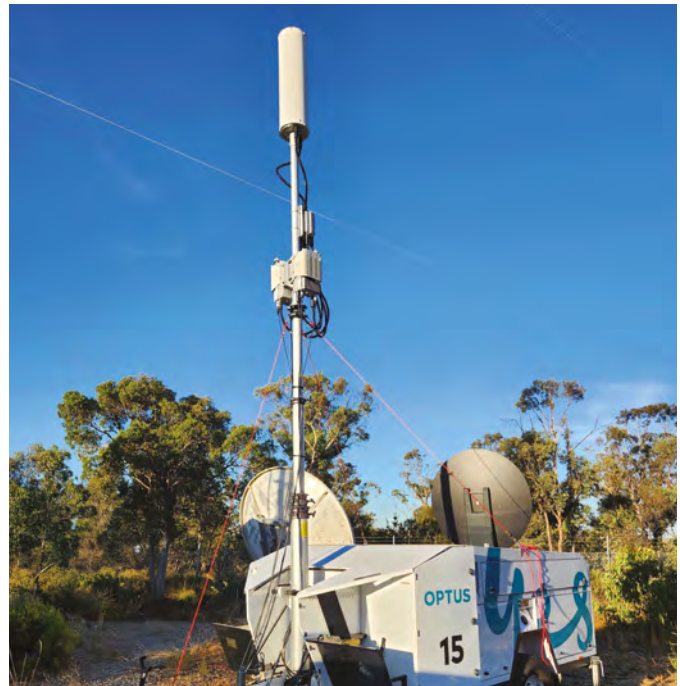
Optus' growing fleet of Cell on Wheels units can be quickly transported and activated to restore mobile services during natural disasters.
