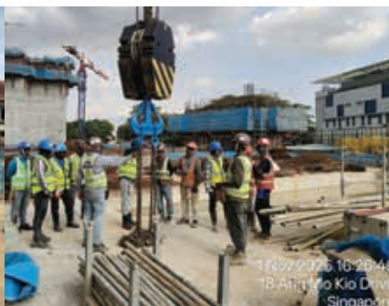
Subcontractors EHS personnel conducting site wide checks ensuring proper checks and balance
