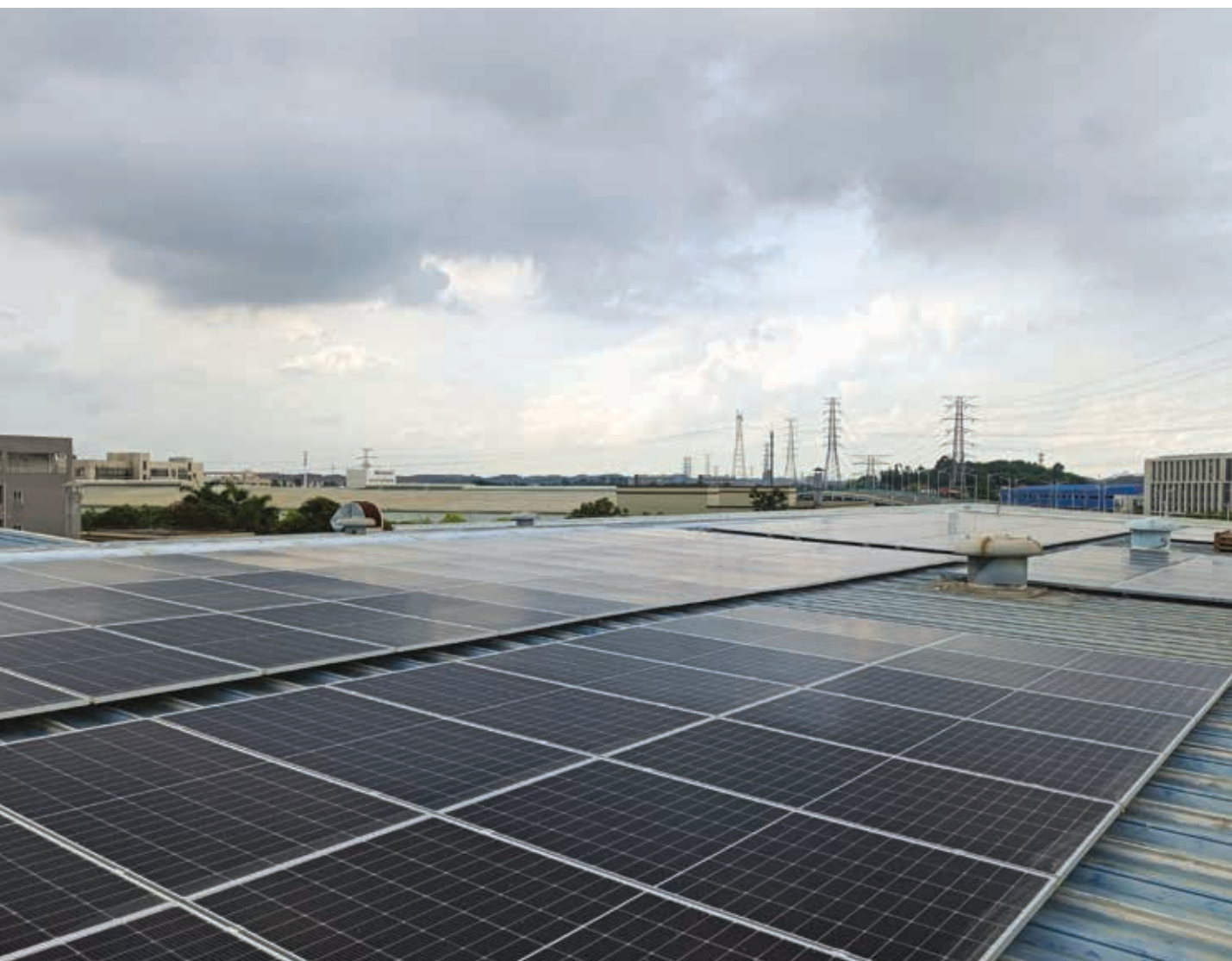
Solar Photovoltaic Panels in China Guangzhou Plant
