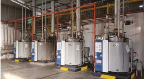
Light Fuel Oil boilers at our Ipoh Plant
