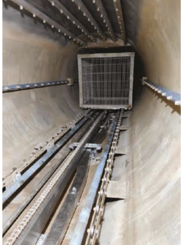
Completion of Retort Low Energy Suction System (LESS) in our China Guangzhou Plant
