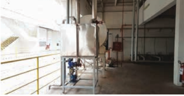
Condensate Recovery System in Cambodia Plant
